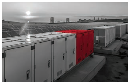
Large Battery Energy
