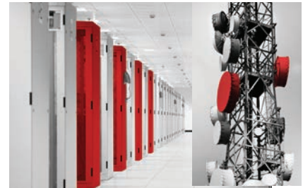
Telecom & Data Center
