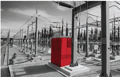
Electrical Sub stations
