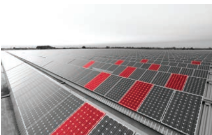
Large Solar Facilities
